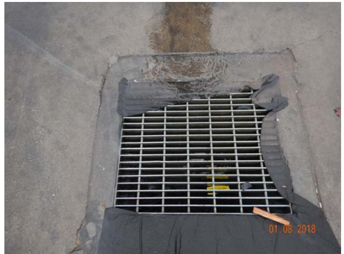
Photo 2. Drop inlet located on the west side of the Facility. All Drop inlets observed with Ultra-Tech Ultra Drain metal-removing BMPs installed.
