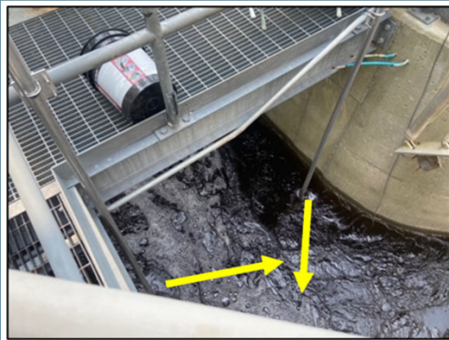
Camera 3&4 - Floor Diffuser
