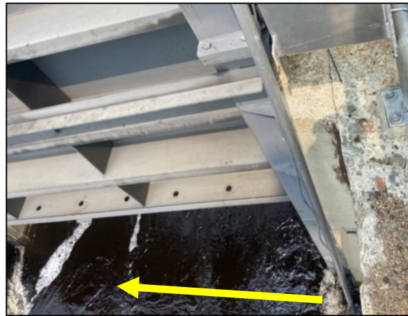
Figure 3. Camera Location 1: Outside of the entrance looking across the flap gate.
