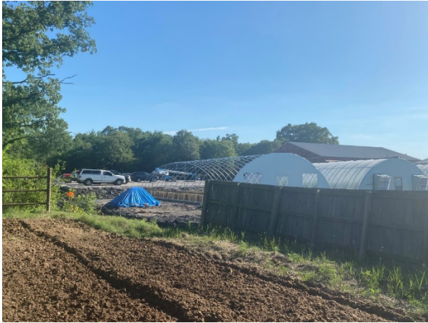
View of construction of the illegal marijuana operation's grow houses from the Grants' property.
