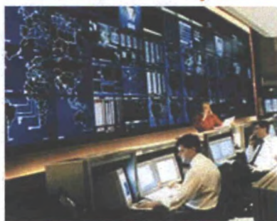
AT&T Network Operations Center, Bedminster, N.J., 1987.
